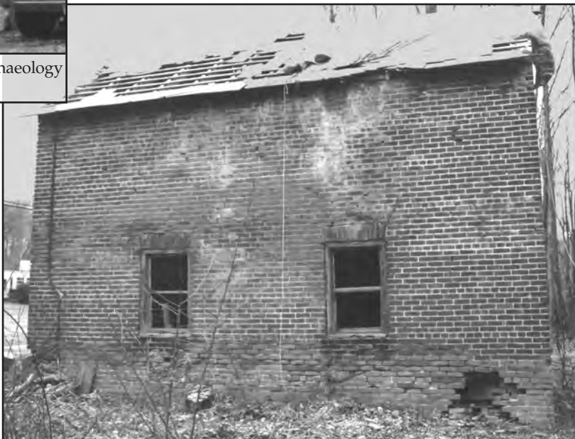
The Whiskey House, January, 1990. With holes in the roof and crumbling masonry, the building was near collapse. PSE&G provided the manpower and material to reinforce the walls. Trees and brush too close to the building were removed.
