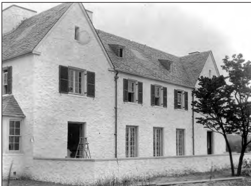
The Lindbergh Estate Under Construction. There were 23 rooms, 6 fireplaces, and 34 closets. The house was built like a fortress, with reinforced concrete floors and stone walls that are 28 inches thick.
